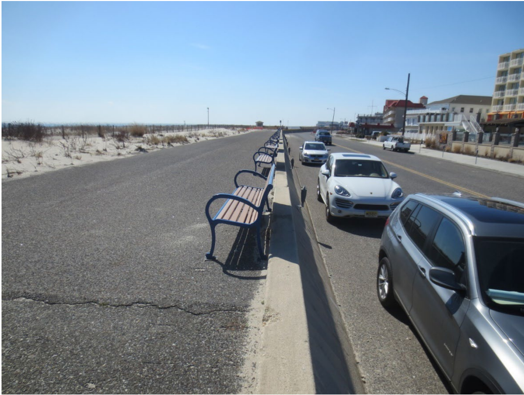
Figure 8: Existing seawall west of Madison Avenue, showing paved top with the concrete wall to the right.
